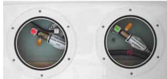
Fuel Valves Aft Tank (Typical)
