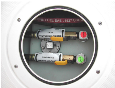
Fuel Valves Forward Tank
