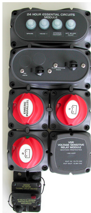
Battery Switches and Main Breakers (Typical)
