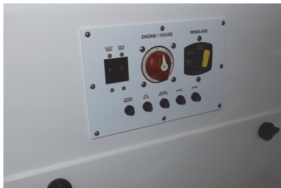
Battery Switches and Main Breakers
