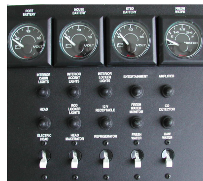
Cabin DC Breaker Panel
