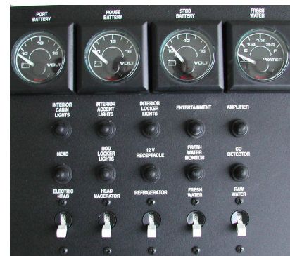
Cabin DC Breaker Panel
