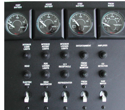
Cabin DC Breaker Panel
