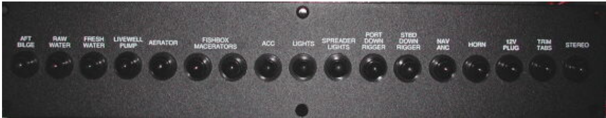
Helm Breaker Panel
