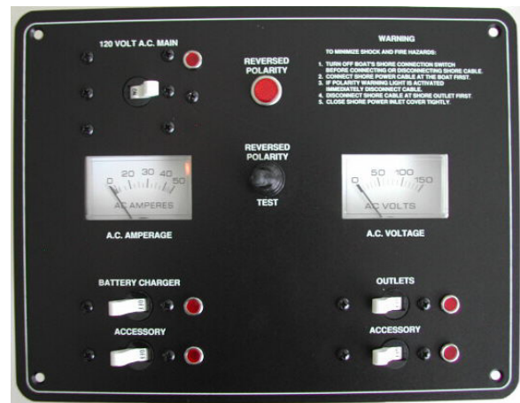
AC Breaker Panel
