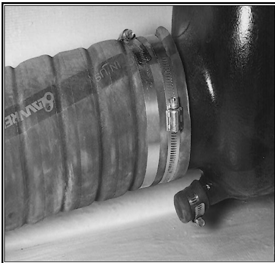
Figure 7-3: Main Engine Muffler
