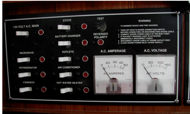
AC Breaker Panel
