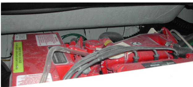
Generator - Upper Access
