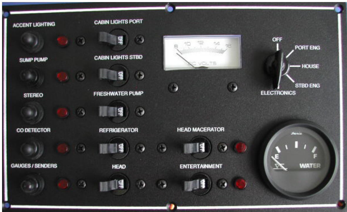
Cabin DC Breaker Panel
