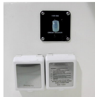
Shore Inlet and Breaker
