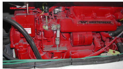
Generator - Lower Access
