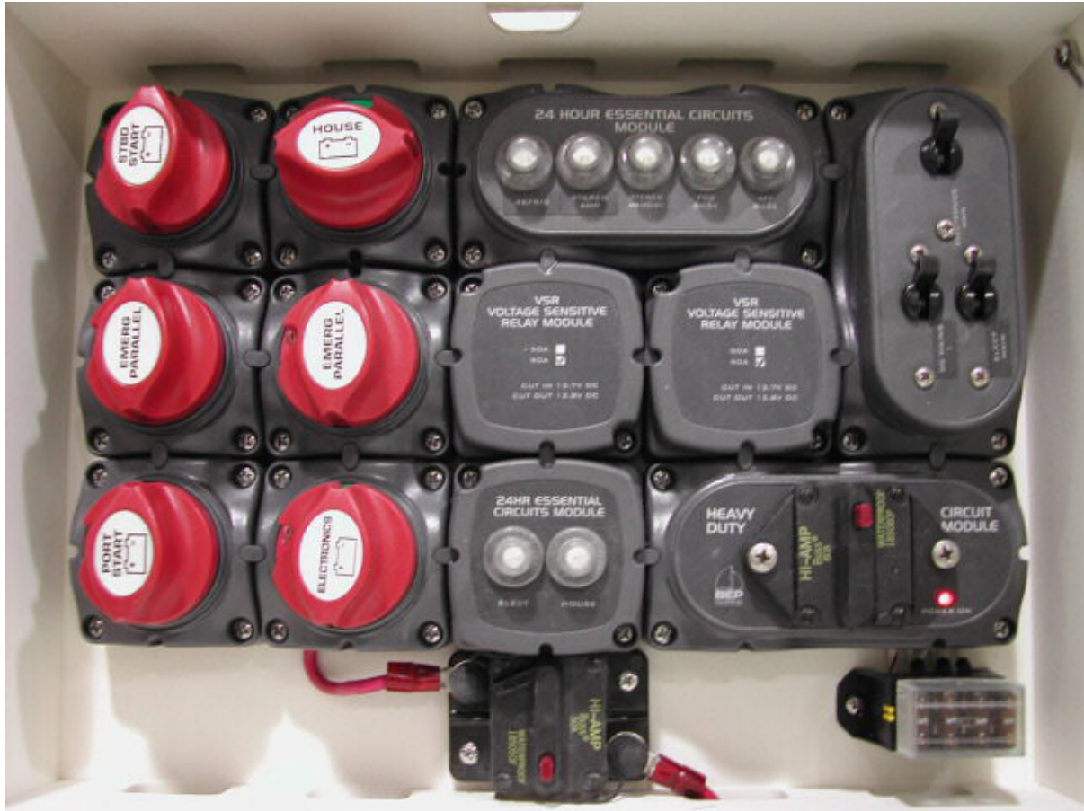
DC Power Distribution
