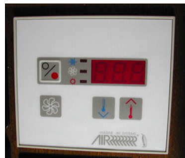
Air Conditioning Control Panel
