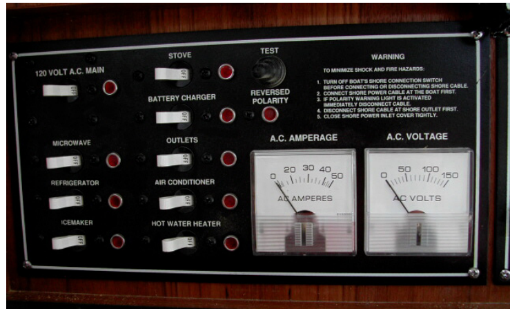
AC Breaker Panel
