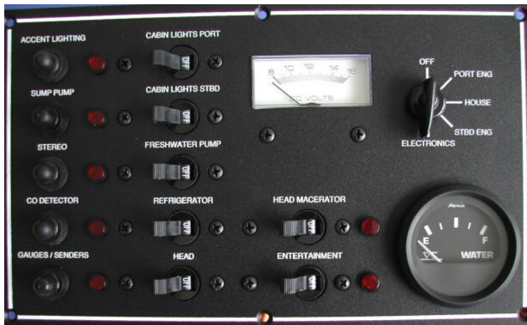
Cabin DC Breaker Panel (typical)
