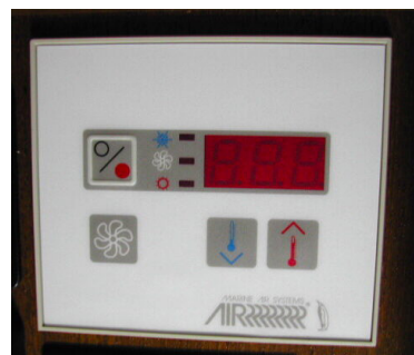
Air Conditioning Control Panel
