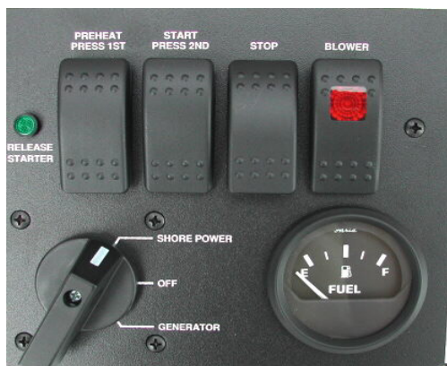
Diesel Generator Panel
