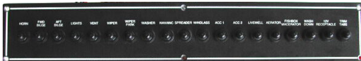
Helm Breaker Panel
