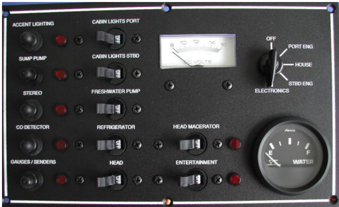
Cabin DC Breaker Panel
