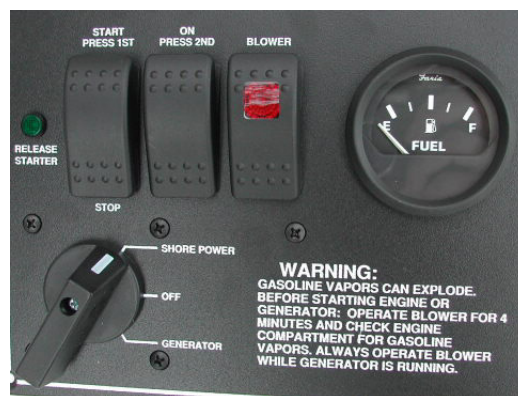
Gasoline Generator Panel
