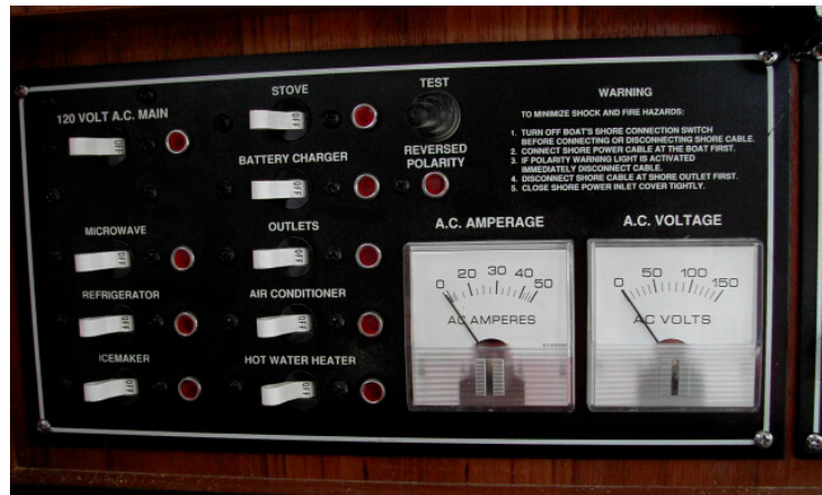
AC Breaker Panel
