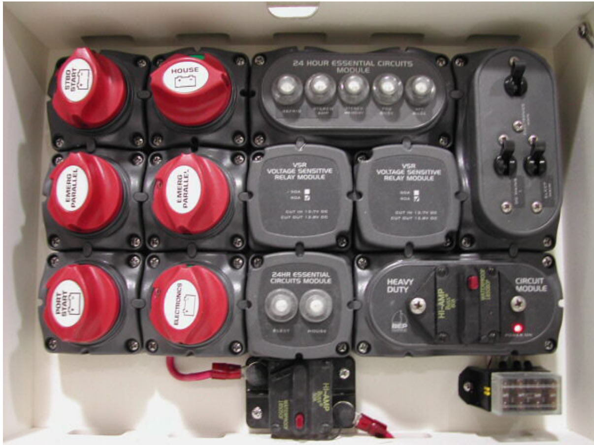
DC Power Distribution
