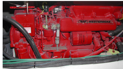
Generator - Lower Access
