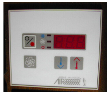
Air Conditioning Control Panel
