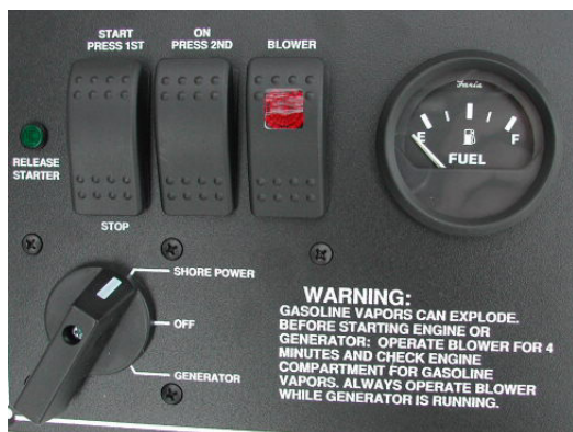
Gasoline Generator Panel
