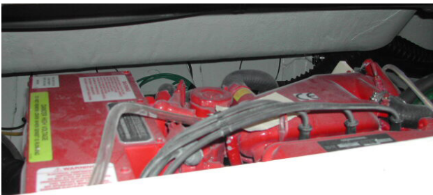
Generator - Upper Access
