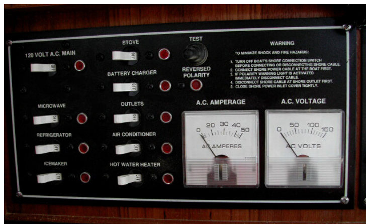
AC Breaker Panel
