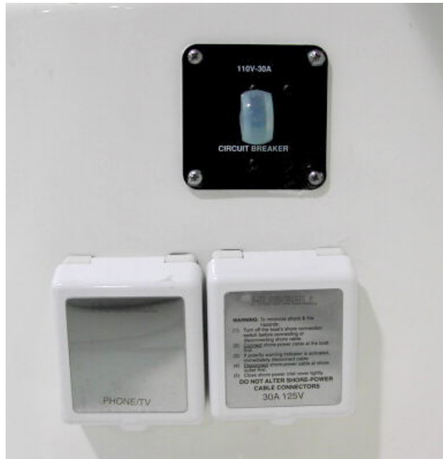
Shore Inlet and Breaker
