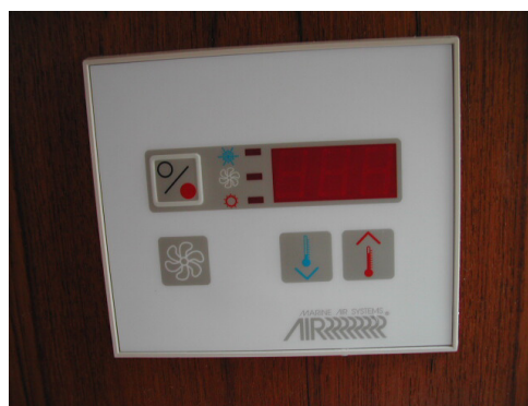
Air Conditioning Control Panel
