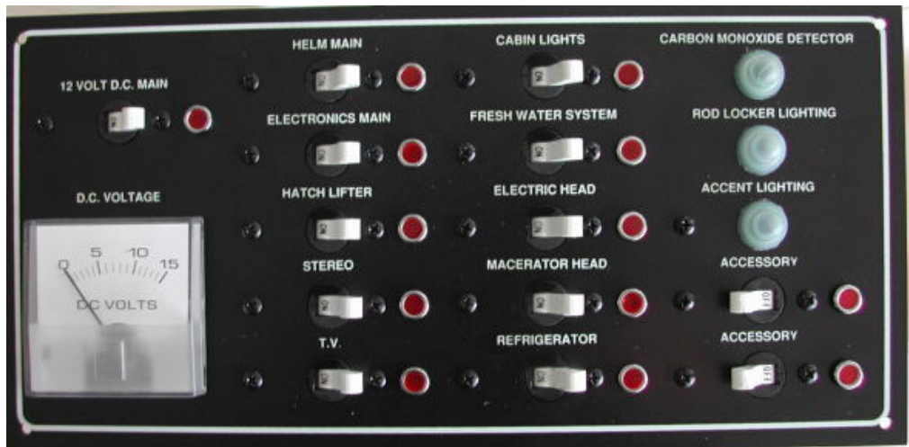
Cabin DC Breaker Panel
