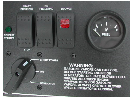
Gasoline Generator Panel
