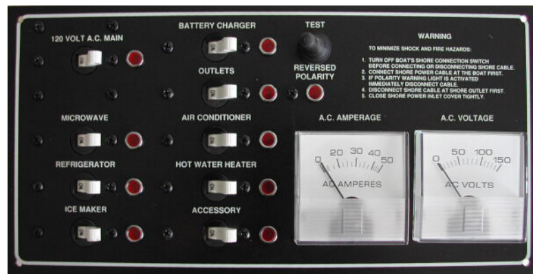
AC Breaker Panel
