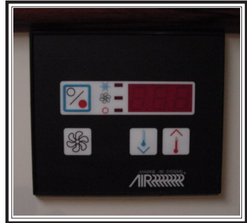
Air Conditioning Control Panel
