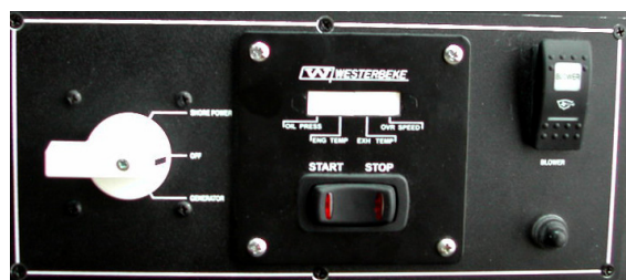
Generator Panel (typical)
