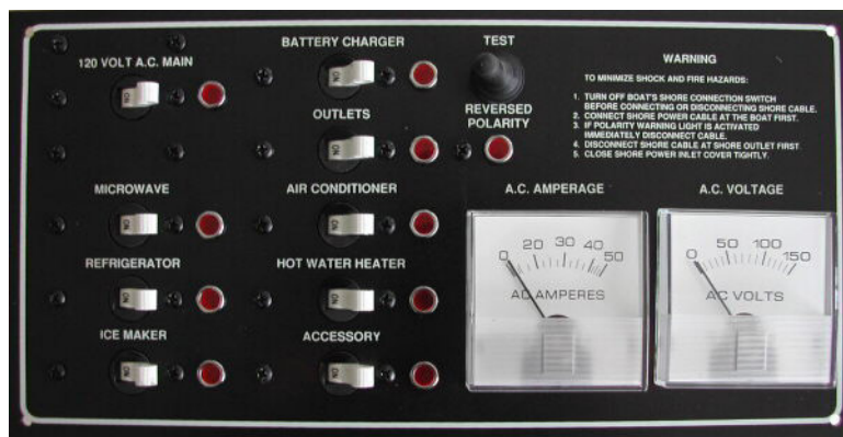
AC Breaker Panel (typical)
