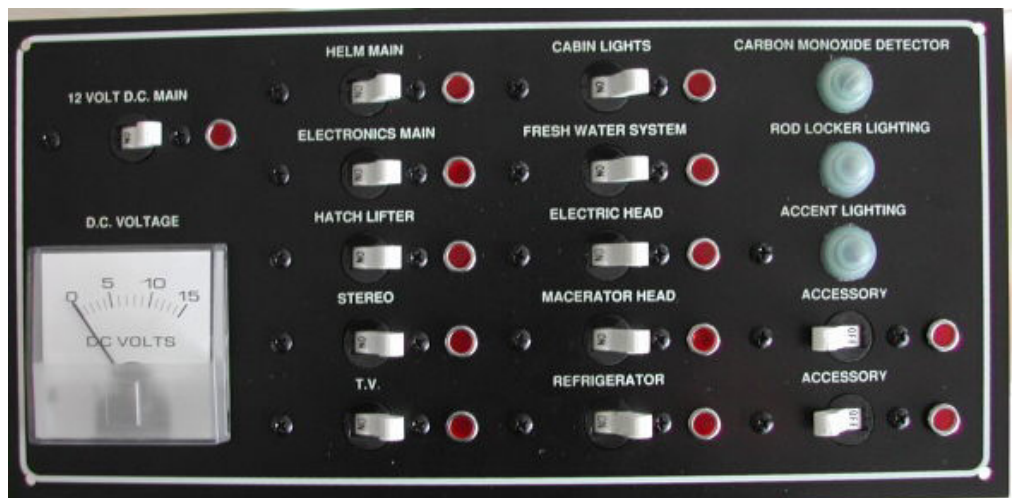
DC Breaker Panel
