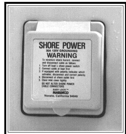
Shore Power Inlet
