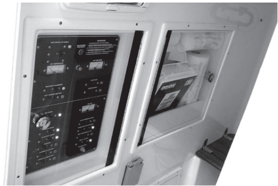
Electrical Panel and Towel Rack
