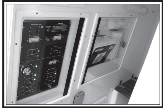
Electrical Panel and Towel Rack
