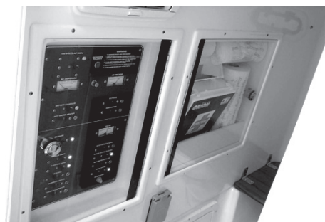
Electrical Panel and Towel Rack
