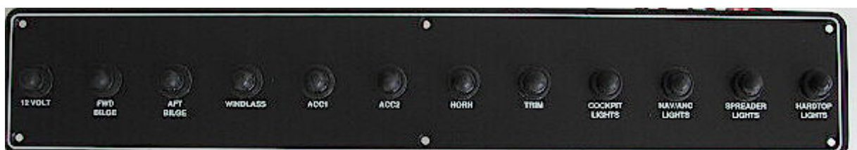
Helm Breaker Panel
