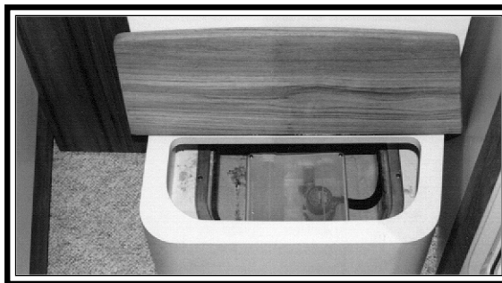
Shower and Cabin Drain Sump Pump
