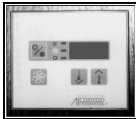
Air Conditioning Control Panel
