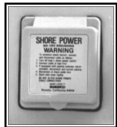
Shore Power Inlet
