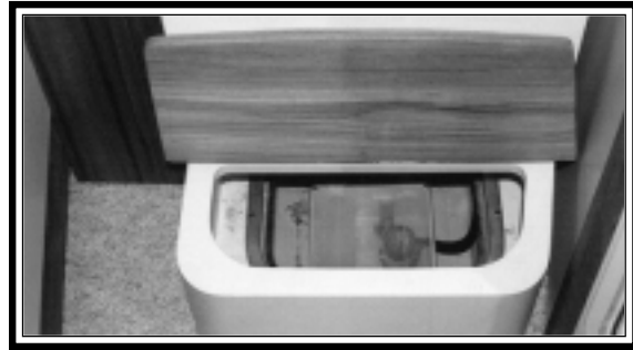
Shower and Cabin Drain Sump Pump
