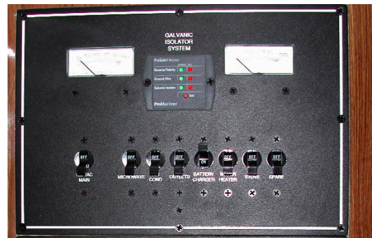
AC Breaker Panel
