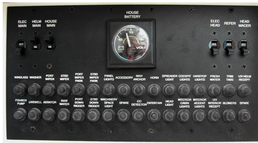
DC Main Distribution Panel (MDP)
