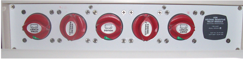
Battery Switch Panel
