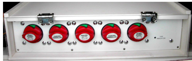
Battery Switch Panel
