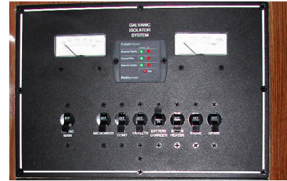
AC Breaker Panel
