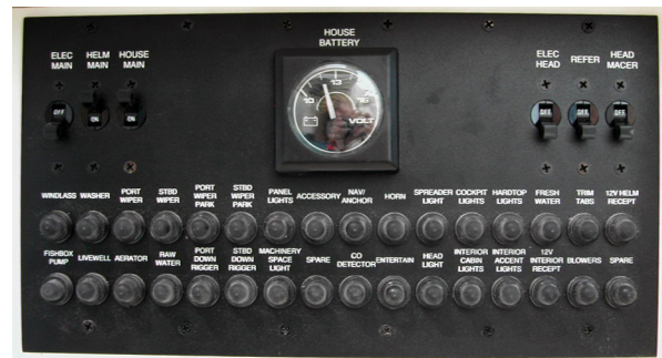
DC Main Distribution Panel (MDP)
