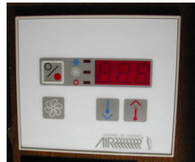
Air Conditioning Control Panel
