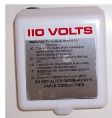
Shore Power Inlet
