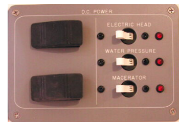
Head Breaker Panel
