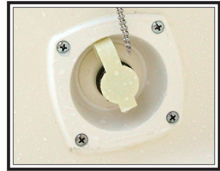
Shore Water Connection
