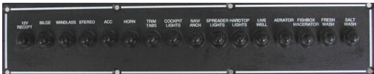
Helm Breaker Panel
