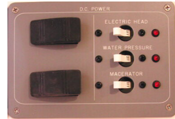
Head Breaker Panel
