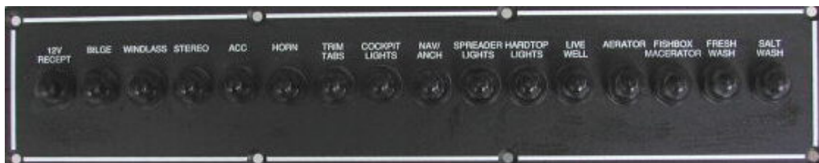
Helm Breaker Panel
