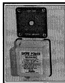
Shore Power Outlet
