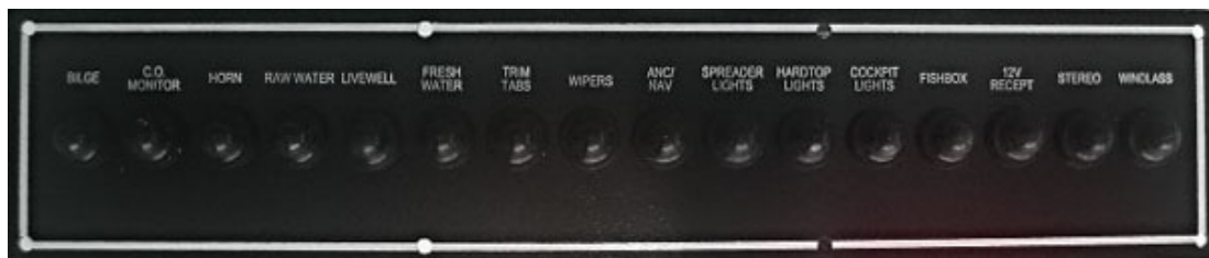
Breaker Panel (typical)
