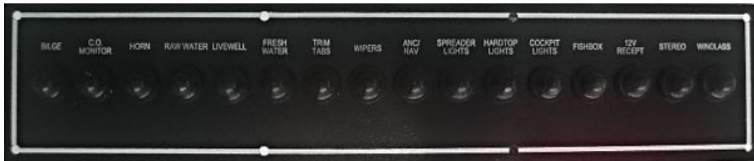
Breaker Panel (typical)
