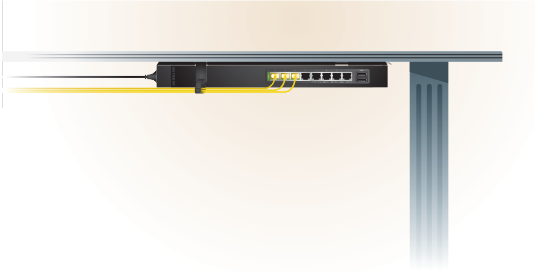
Figure 13. Cables strapped to the bracket
