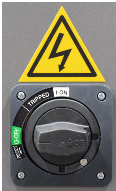
Main power isolation switch
