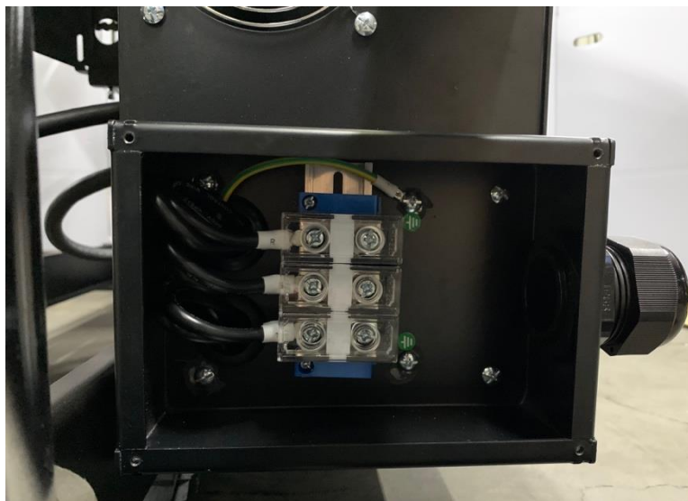
Figure 11: Electrical Connection Box
