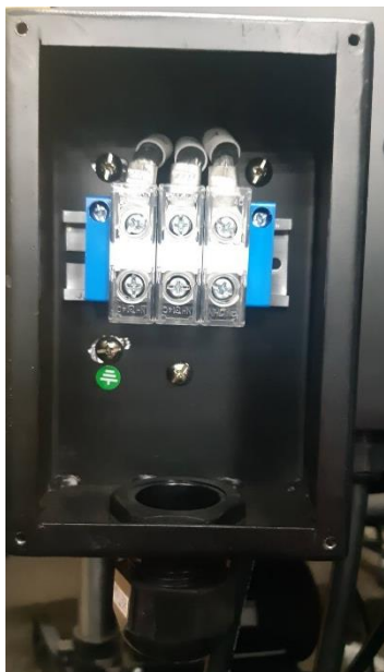
Figure 11: Electrical Connection Box
