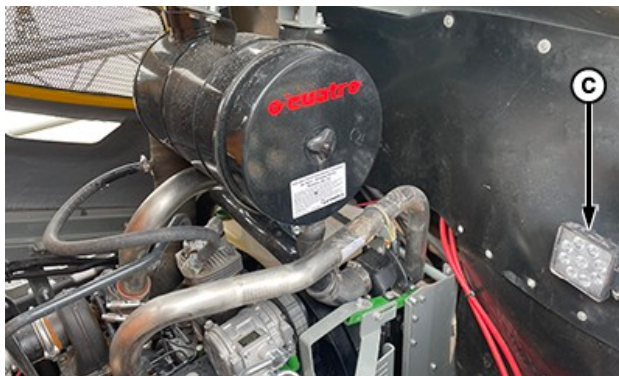
Square Maintenance Lights—Engine (One at each engine side)
