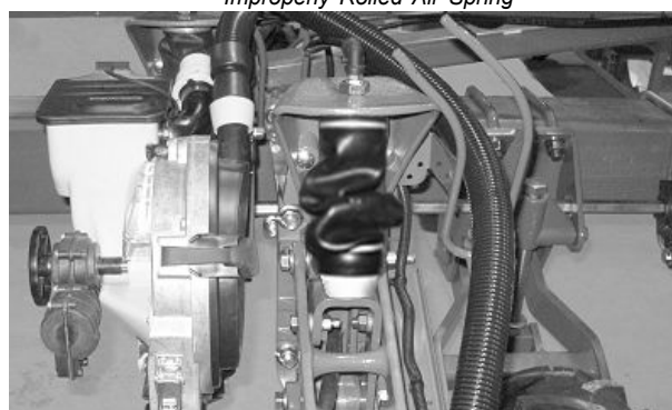
Improperly Rolled Air Spring (Twin Row)
