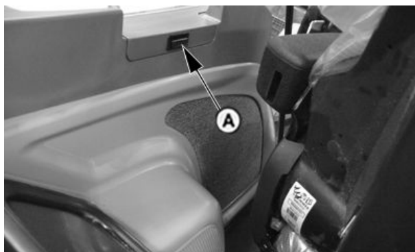
Main Fuse and Relay Load Center (Left Console)
