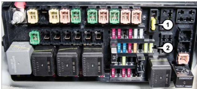
Power Outlet Fuses
